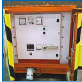
Figure 4, typical 550V LV panel, with IP 23 rating
