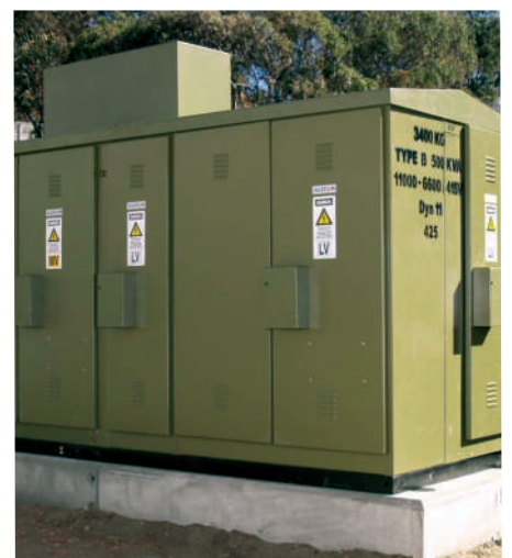
Miniature substation with IAC.
