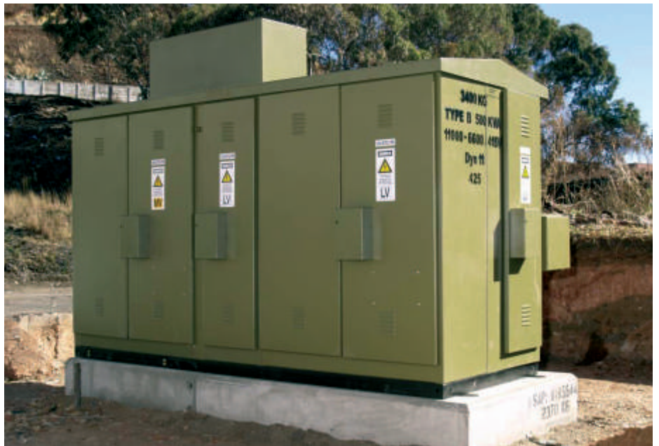
Miniature substation with IAC.
