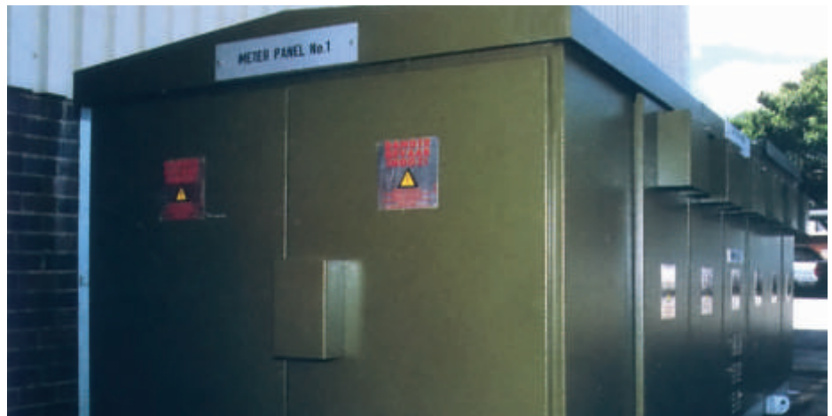
Rhino outdoor substation.
