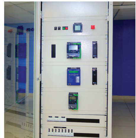
Protection and control panel
